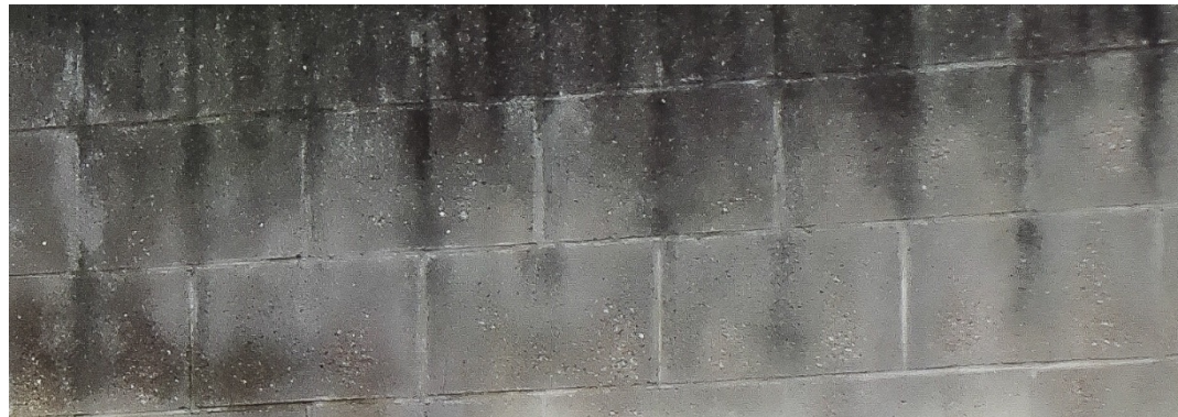
Mold on wall
